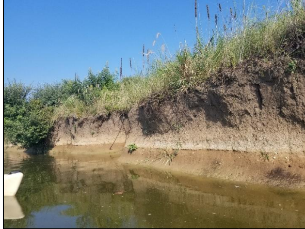
Figure 12: Bank erosion along Ewing Island.
